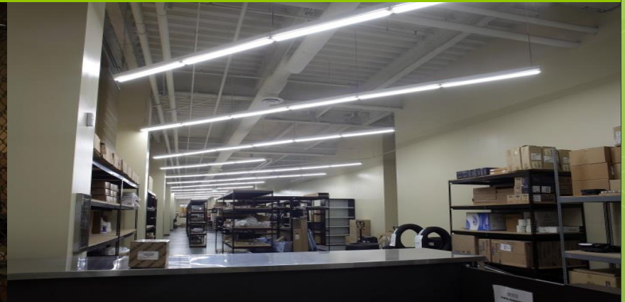
After – 16W LED T8 Retrofit
