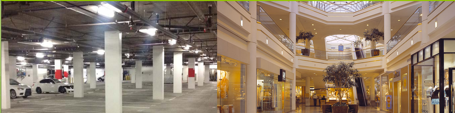
AFTER – LED Can Retrofits & Bi-Level Parking Fixture
