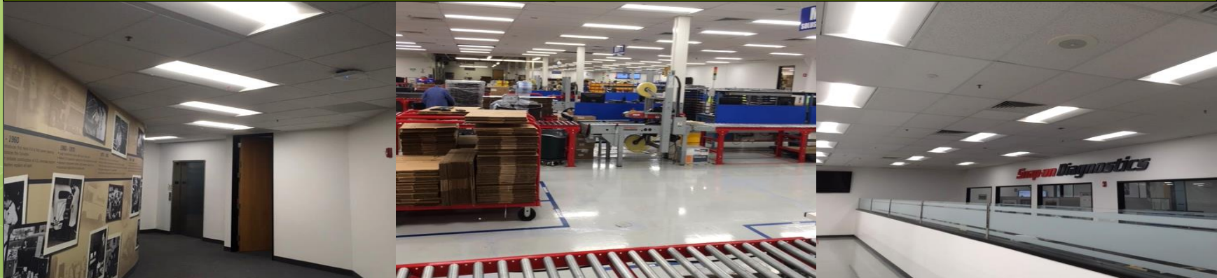
After: LED Troffer Retrofit
