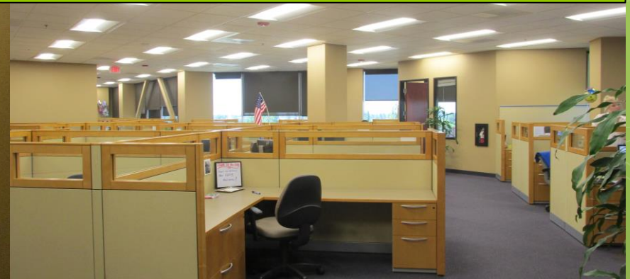
AFTER – 30W LED Troffer Retrofit KUDO
